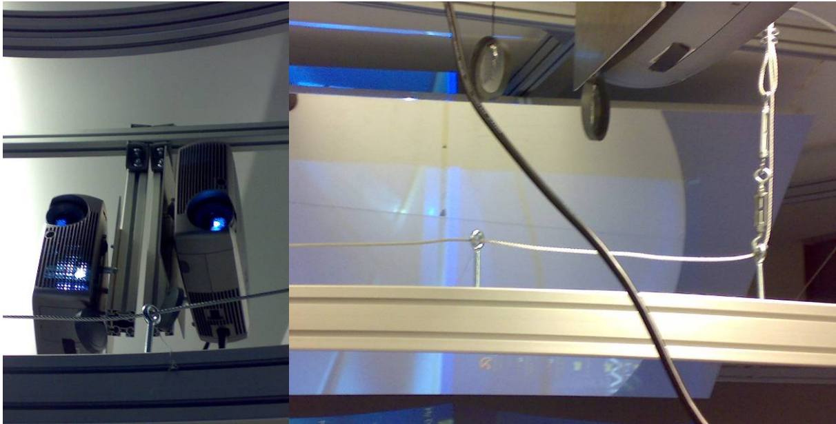
Fig. 7) Attachment of the ceiling projectors and mirrors
